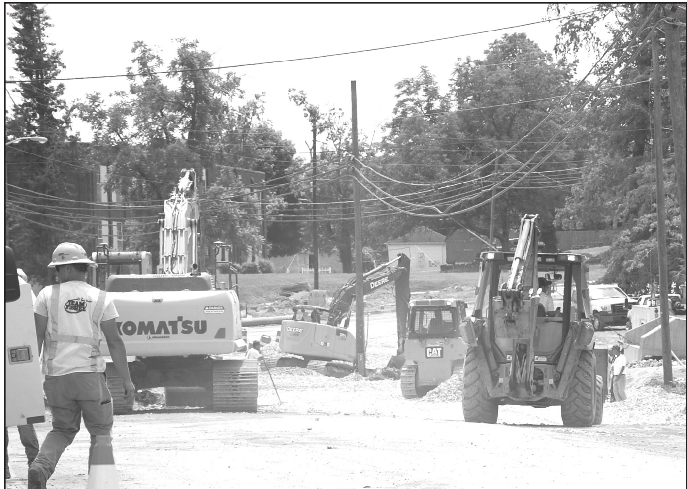
Work continues on the Sweet Lick Creek Bridge near the Estill Springs School on the north end of Irvine as part of the re-construction of KY-89 North, Winchester Road. The road has been closed for over a week but is expected to reopen on Thursday, July 21st.
