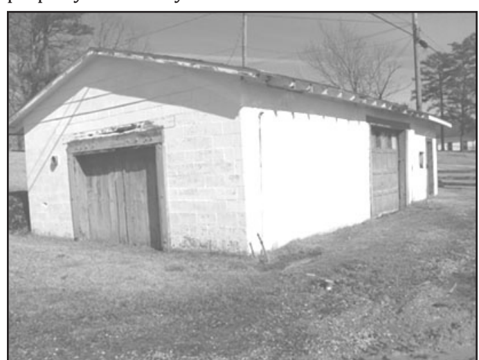
The garage as it appears today. It has been vacant for several years.
