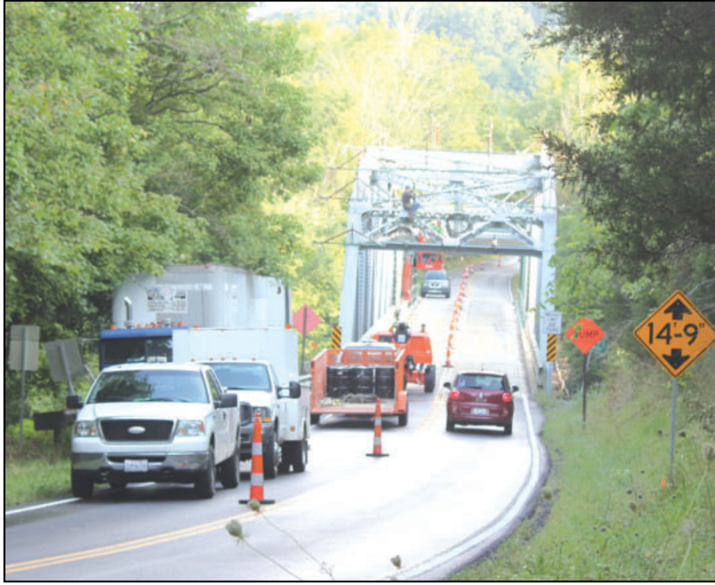
The painting of the bridge on the Clark and Estill County line on Highway 89 has resumed. While the bridge is being repainted, there is a traffic light on each side of the bridge. The three miles of the Winchester Road which had breaks-in pavement were repaved recently.
