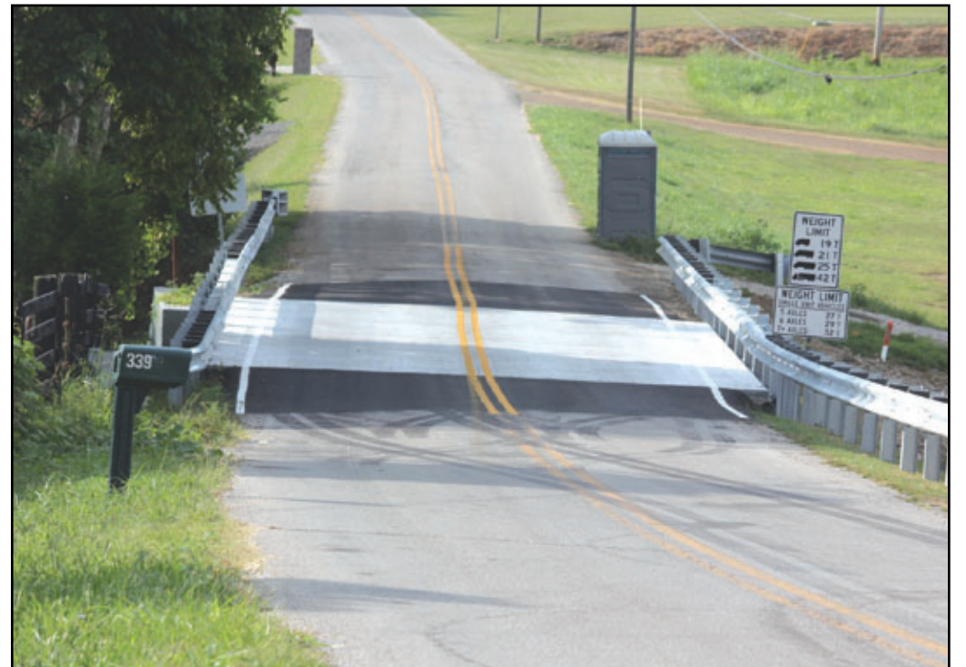
Dry Branch Road reopened to traffic several weeks ago after it was closed while the bridge over White Oak Creek was replaced. Tonnage signs for trucks are in place for the bridge. It was one of the bridges on the state's replacement list.
